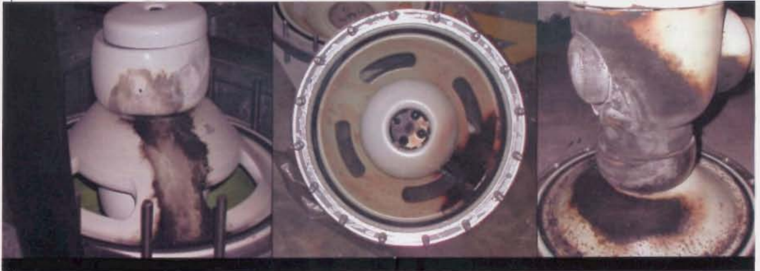
Fig. 2. Examples of faults due to flashovers at insulating surfaces when the SF 6 quality has degraded.
